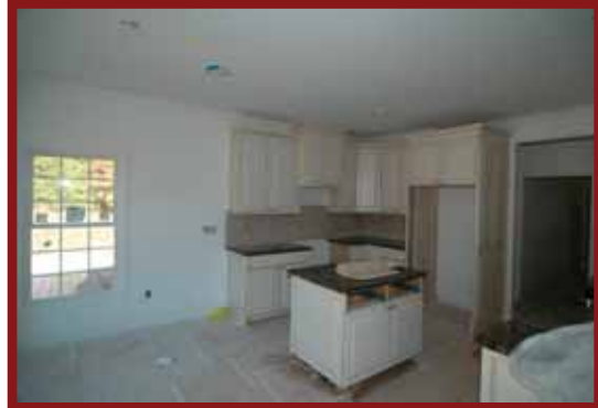
Granite Counters & Upgraded Cabinets
